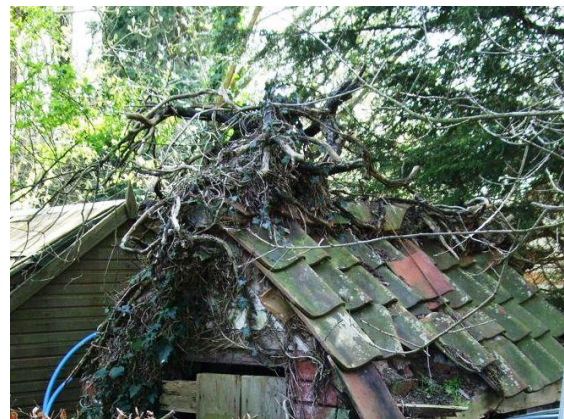
Figure 33 Clay pantiles are found on many outbuildings including this small building in the grounds of The Old Victoria
