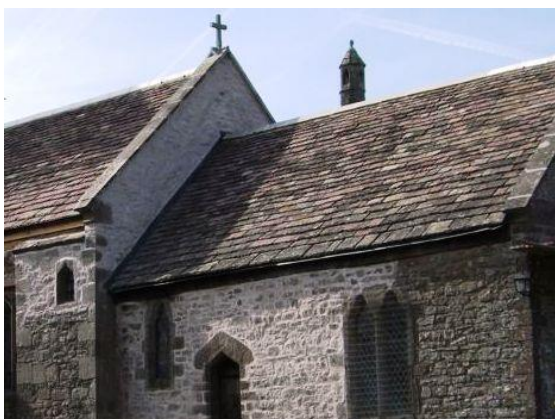
Figure 32 Stone slates are a feature of St John's church. These are traditionally laid in diminishing courses which gives a very attractive highly textured roof finish
